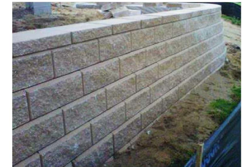
retaining walls to east side of site - allan block with geogrid reinforcement
